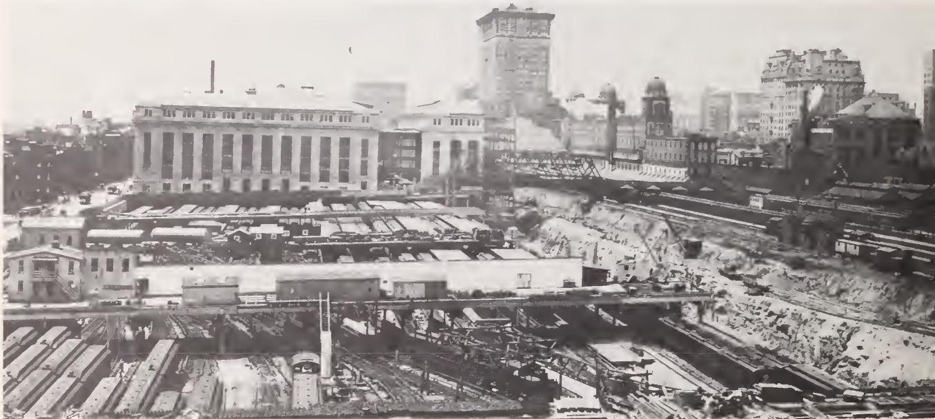
Fig. 11. New marshalling yards, Grand Central Terminal. This 1909 photograph shows the extraordinary ways in which new tracks, platforms and station house were constructed without interruption to service over 600 local and long-distance trains per day.
